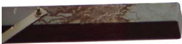
This fibreglass composite cross arm is evident of tracking from leakage currents after service in a coastal application
